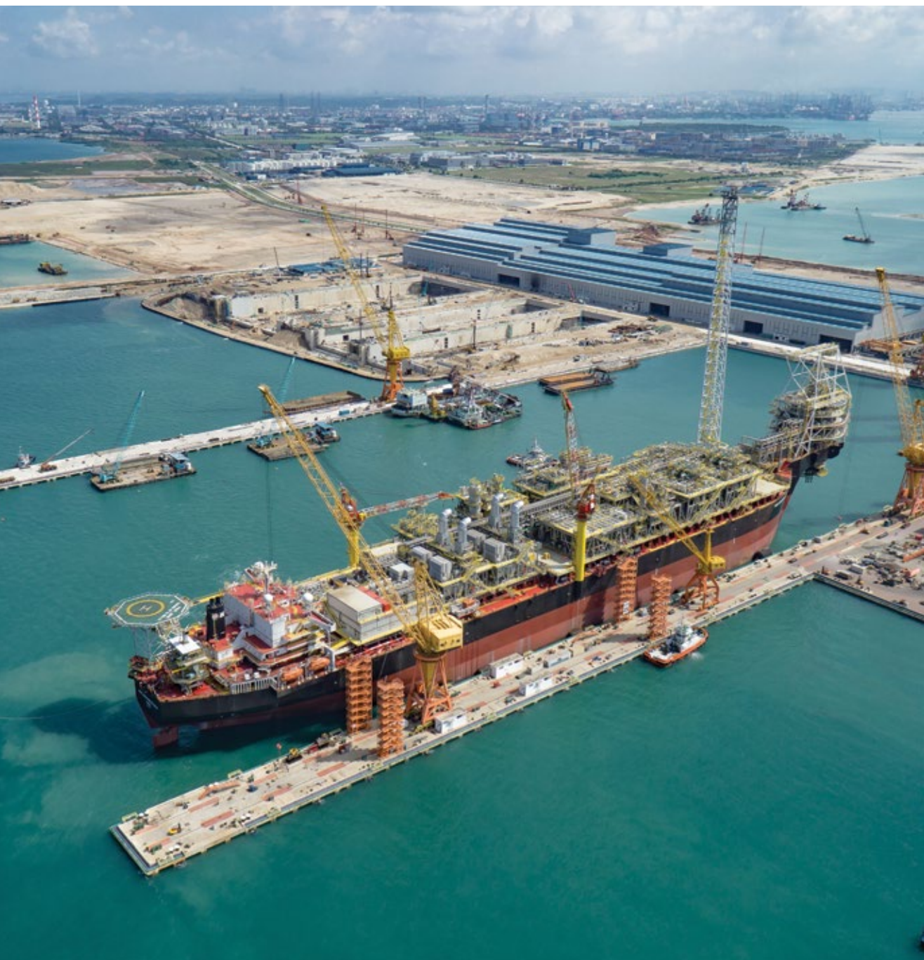
Phase II of the state-of-the-art Sembcorp Marine Tuas Boulevard Yard in Singapore, expected to be completed in 2017
